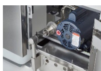
8 gpm filter pump
